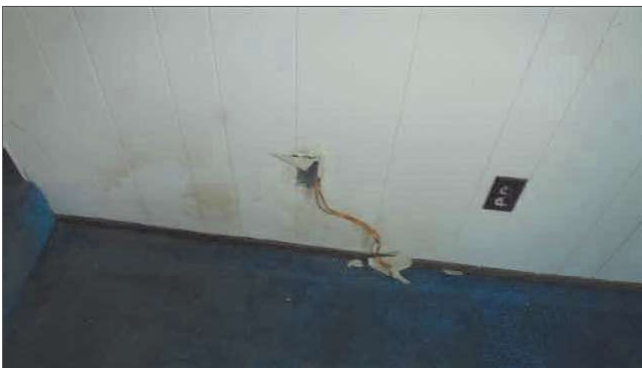
7.1 (3) This junction box is missing a cover.
