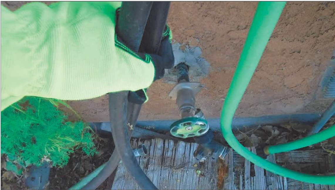
6.1 (1) The water supply, distribution and fixtures were inspected. Most water distribution pipes were not visible due to wall, floor and ceiling coverings. Hose bibs on the exterior are not attached to the wall using the mounting flange.
