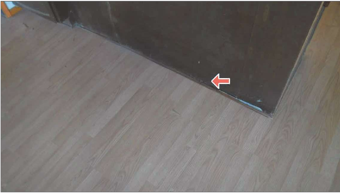
4.3 (3) Trim is damaged on this cabinet.
