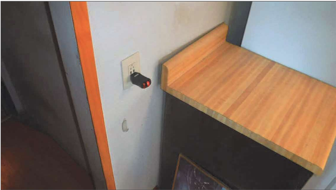
7.1 (2) This receptacle had an Open Ground condition. This condition should be corrected by qualified electrical contractor.
