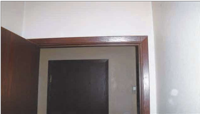
4.4 (3) This interior door rubs when opening and closing it.
