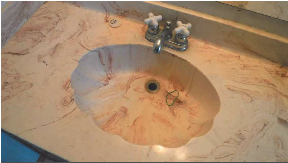
6.0 (1) The plumbing drain, waste and vents were inspected. The drain stopper is missing from this plumbing fixture
